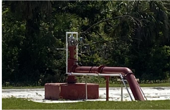
Photo 4-2: Existing Deep Injection Well
